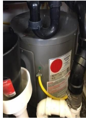
Tank water heater
