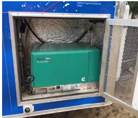
Generator installed in exterior compartment of unit
