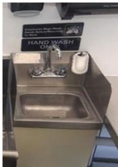
Fixed standalone handwash station
