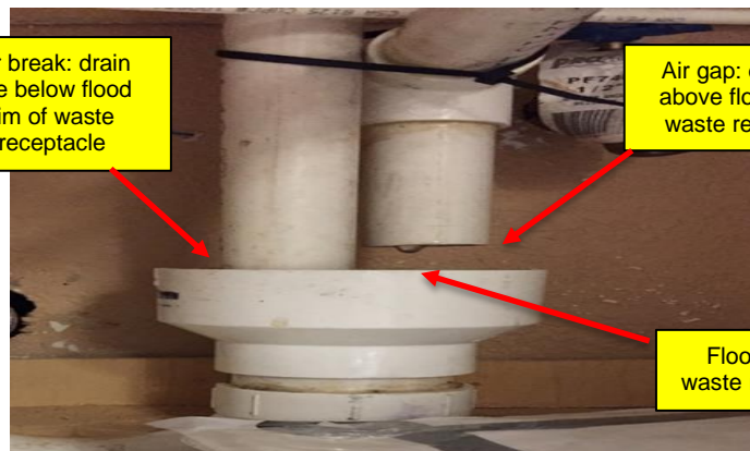
Indirect connection (air gap or air break)- permitted on equipment in which food, portable equipment or utensils are placed. Drainline off ice bins/machines must be through an air gap.
