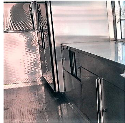
Equipment sealed to each other, floor, and back wall to prevent debris from accumulating underneath, behind and between equipment.
