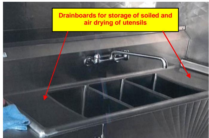
Fixed 3-compartment set up with drainboards
