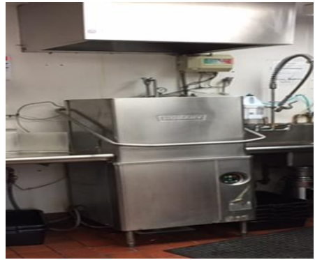
Type II hood over heat/moisture producing dishmachine
